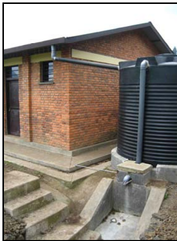
Figure A-7: New tank at primary school
